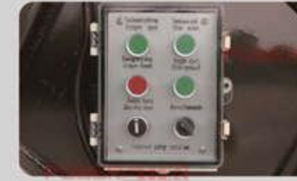
Germany SIEMENS PLC control box
