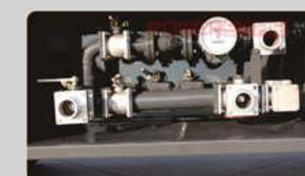
valve system with flow meter
