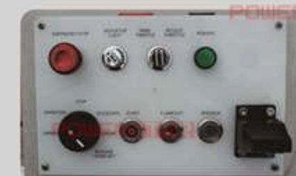
PLC control box in cage
